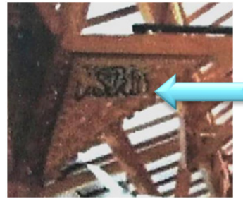
Picture 21. The main structure of the roof using exposed wood and the application of carved ornaments. (Source : Author, 2020)
